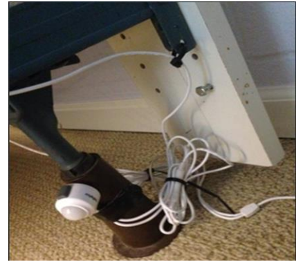
Figure 19: The wires were much too long. The installer had to use multiple zip ties and gorilla tape to manage the cords.
